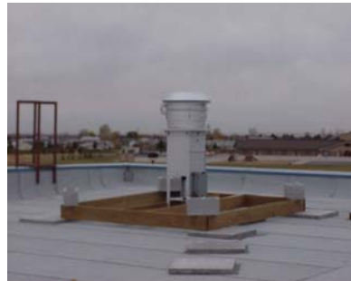
PM 10 Monitoring Equipment
