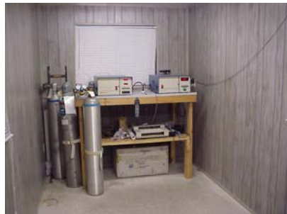
Nitrous Oxide (NOX) Monitoring Equipment
