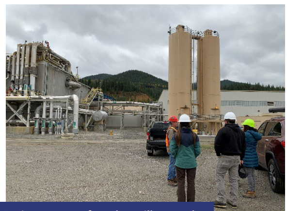
DEQ gives a tour of Bunker Hill Central Treatment Plant, which treats mine water and groundwater to remove metals to improve water quality in the South Fork Coeur d’Alene River.
