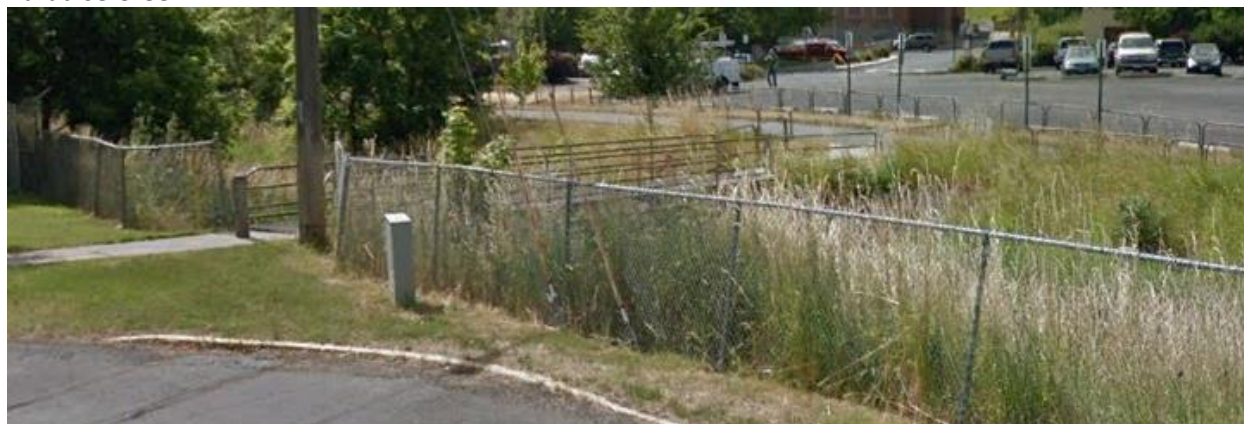
The existing Pedestrian Bridge at the southern extent of Home Street. The bridge deck is too narrow, sits too low within the flood plain, and handrails/guardrails are not compliant and unsafe.
